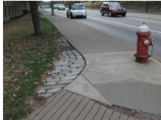
Photo 4 - Northeast corner of Morewood at Forbes Avenue. The landing area for wheelchair occurs over block stone and grass. The block stone is utilized in numerous places along Forbes Avenue in an attempt to widen pedestrian pathways. The area settles and subsequently becomes filled with silt and standing water during rains and ice in freezing weather.
