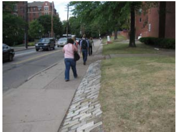
Photo 7 - This photo was taken along Morewood Avenue the major access route to dormitories and fraternity houses. Not only is no buffer afforded here, but pedestrian couples passing in opposite directions, a common occurrence, cannot pass each other. Therefore, on occasion pedestrians will step in the street to pass.
